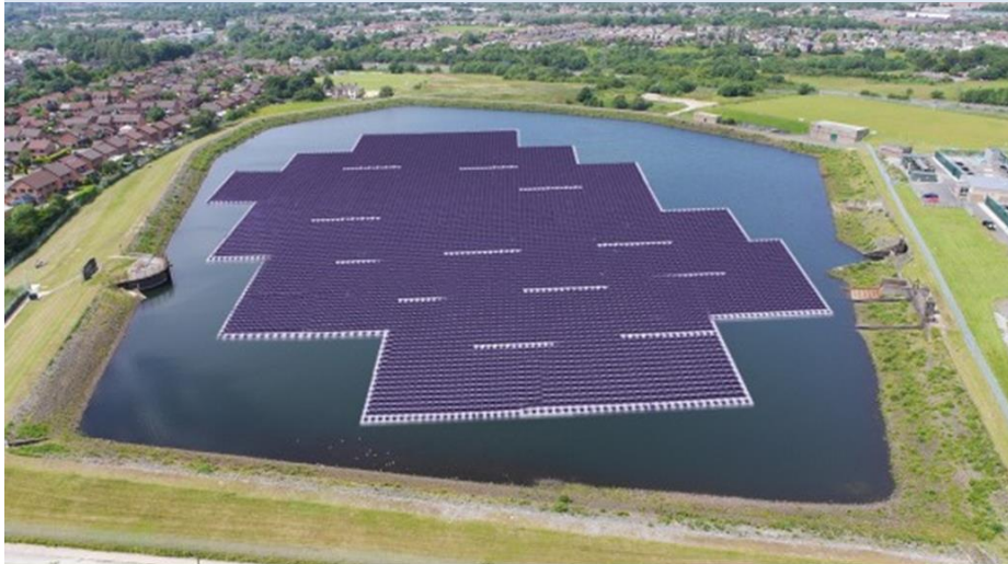
~3 MW floating PV in Hyde, Manchester (UK, 2.7 GWh) 12,000 panels, 45,500 m 2 floating area, 60,000 m 2 lake
