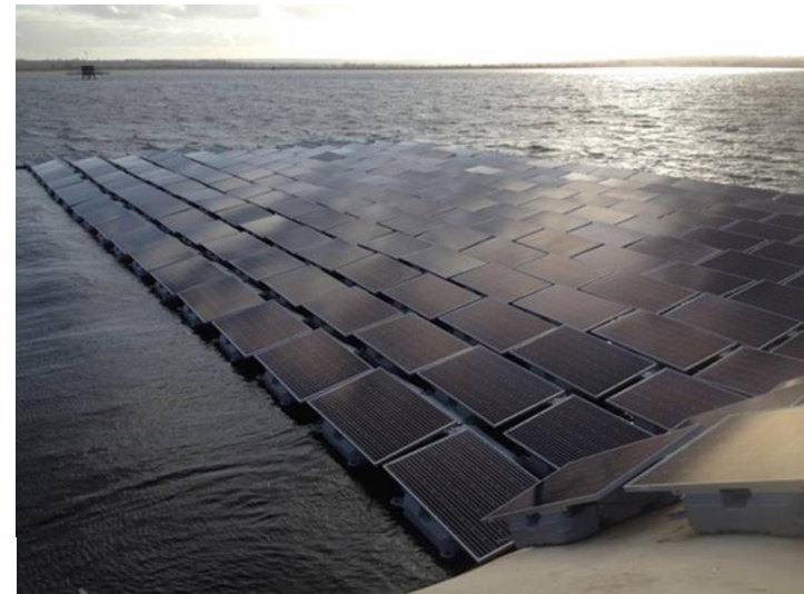
6.3 MW floating PV in London, Queen Elizabeth Reservoir (5.8 GWh)
